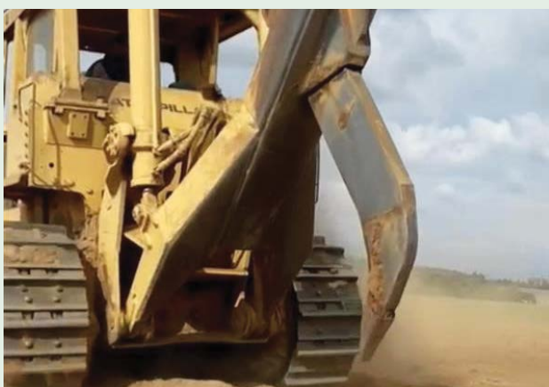
The ground preparation includes breaking up the clay pan which sits at 1.5m to improve drainage in the orchard, and prevent Kiwifruit Vine Decline Syndrome (KVDS).
